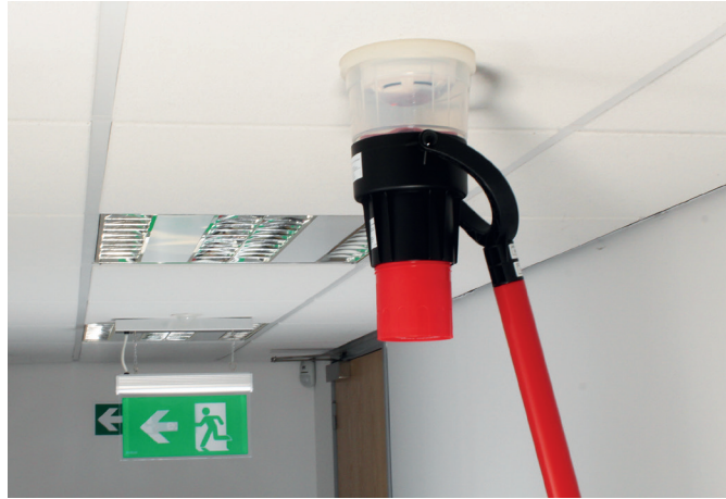
A smoke alarm being tested with an ionisation tester.
