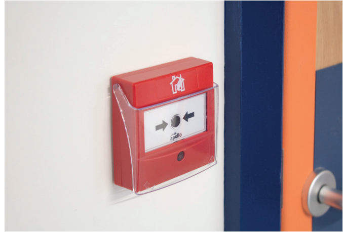
A manual call point which will activate a fire alarm when the glass is broken.
