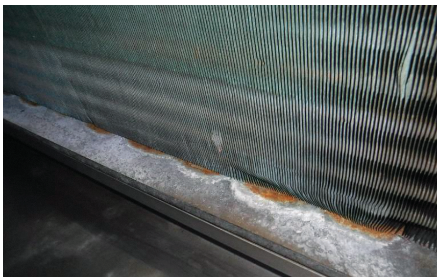
Figure 2: Rust at the base of a frost/fog coil.
