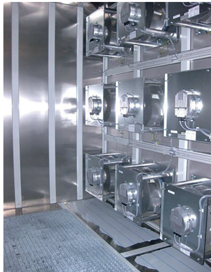
Figure 3: A fan wall in situ .
