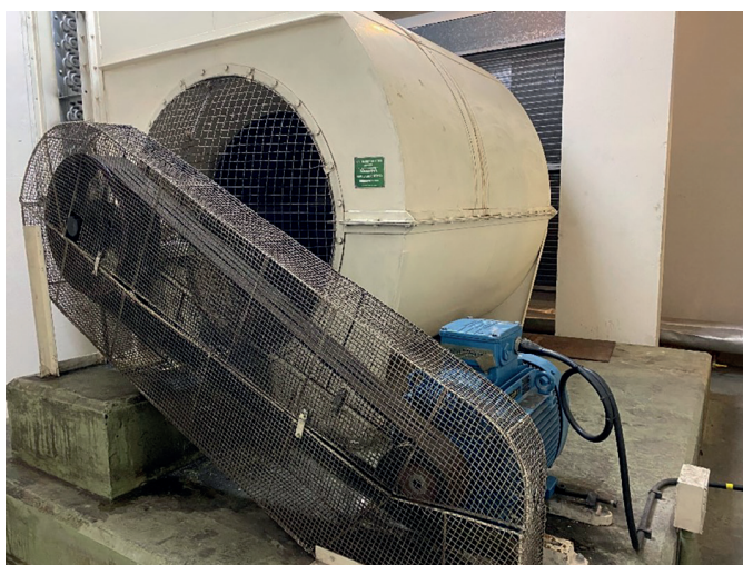
Figure 2: A large legacy belt-driven fan that could be replaced by a fan wall.
