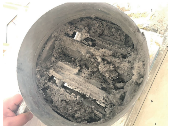
Figure 4: A heavily loaded duct.
