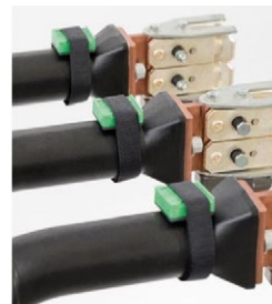
Connection Temperature Monitoring
